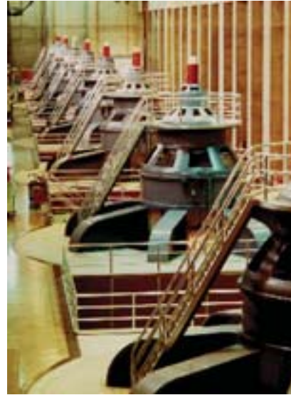
A series of hydel generators.
