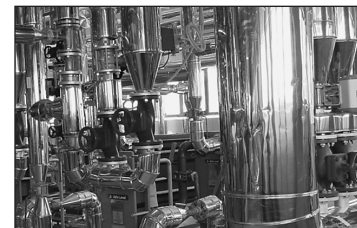
Industrial applications Courtesy UMDE Engineering, Contracting, and Trading. Used by permission.
