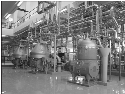
FIGURE 8–41 A piping network in an industrial facility.
