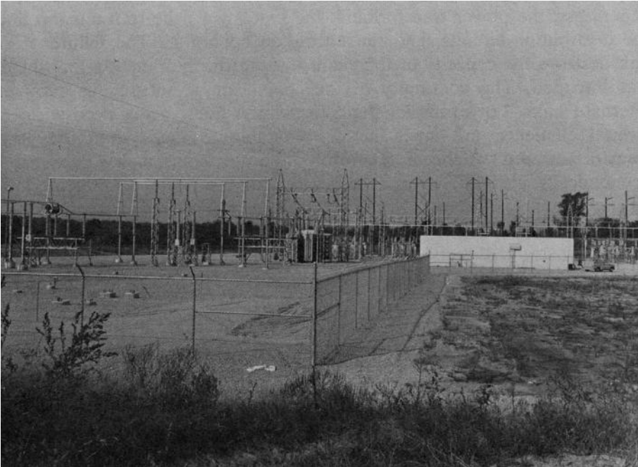
FIGURE 7.2 Typical 345/138-kV transmission bulk-power station. (Courtesy of Union Electric Company.)
