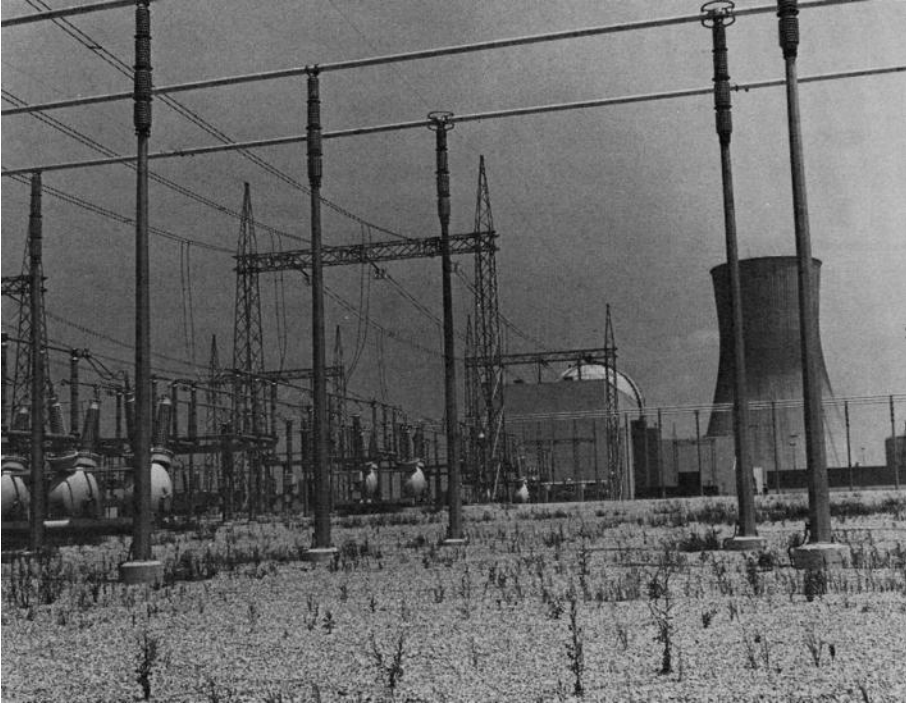
FIGURE 7.1 Callaway nuclear power plant switchyard. (Courtesy of Union Electric Company.)
