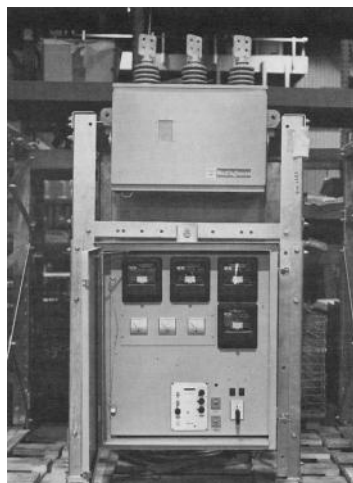
FIGURE 7.6 Typical three-phase automatic circuit recloser. (Courtesy of Union Electric Company.)
